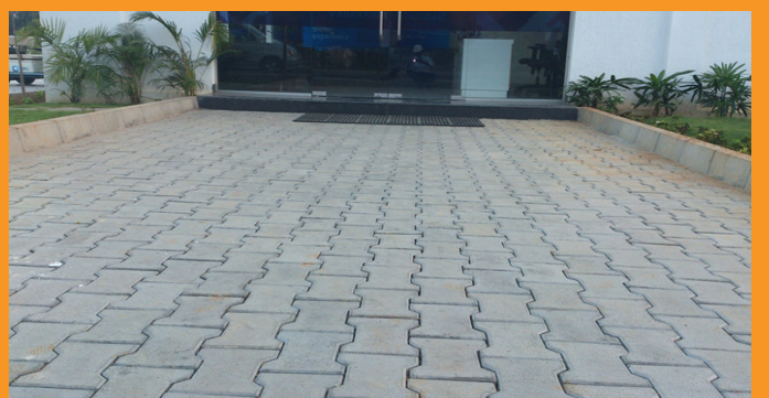
INTER LOCKING PAVER BLOCK WORK AT PBEL CITY, THAYUR, KELAMPAKKAM, CHENNAI – OMR
